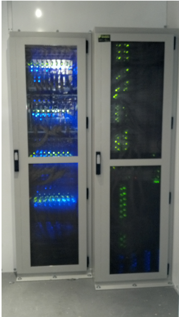
FIG. 5.— Front view of LEDA correlator racking (right). Large-format EMI air filters adopted to enable most readily the front-back airflow required by the digital hardware comprise the door. Screening at 40 MHz is \sim 50 dB. The lefthand rack contains high-gain analog electronics and is independently shielded against RF interference. RF-tight pass throughs in the common wall convey signals from the analog electronics to the correlator digital samplers. The setup is conceptually similar to that adopted for LWA1 (Taylor et al. 2012; Ellingson et al. 2013) though more compact and capable of supporting greater power and computational density.
