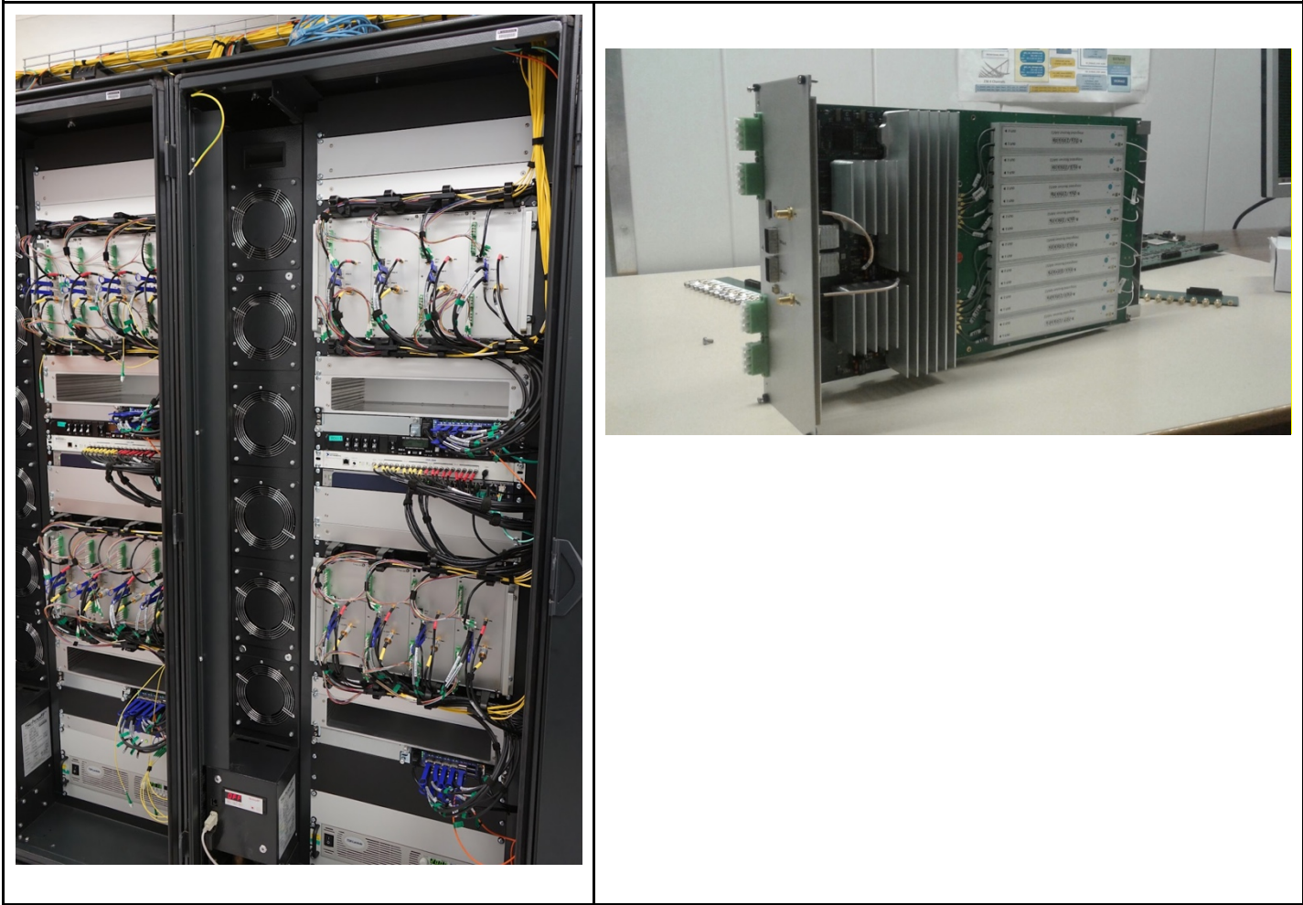
Figure 3; The Signal Processing Cabinet and a Tile Processing Module (TPM) on the right
