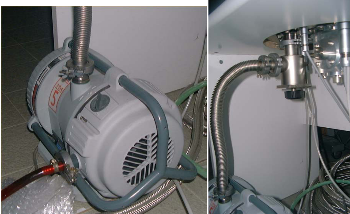
Fig. 3 Vacuum dry pump Boc Edwards XDS5 (left) and connection to the facility by its valve (right)
