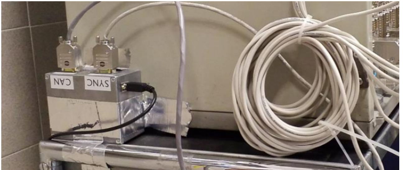
Figure 27 External SYNC/CAN box (temporary backup for the CAN/SYNC board)
