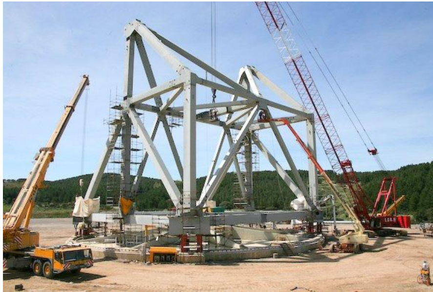
Fig. 1: Photo at the SRT site showing the status of the telescope construction work (May 2008).
