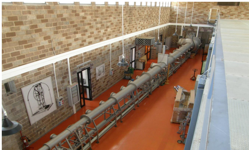
Fig. 10: View of the 35 m long XACT facility, at INAF/OAPA.
