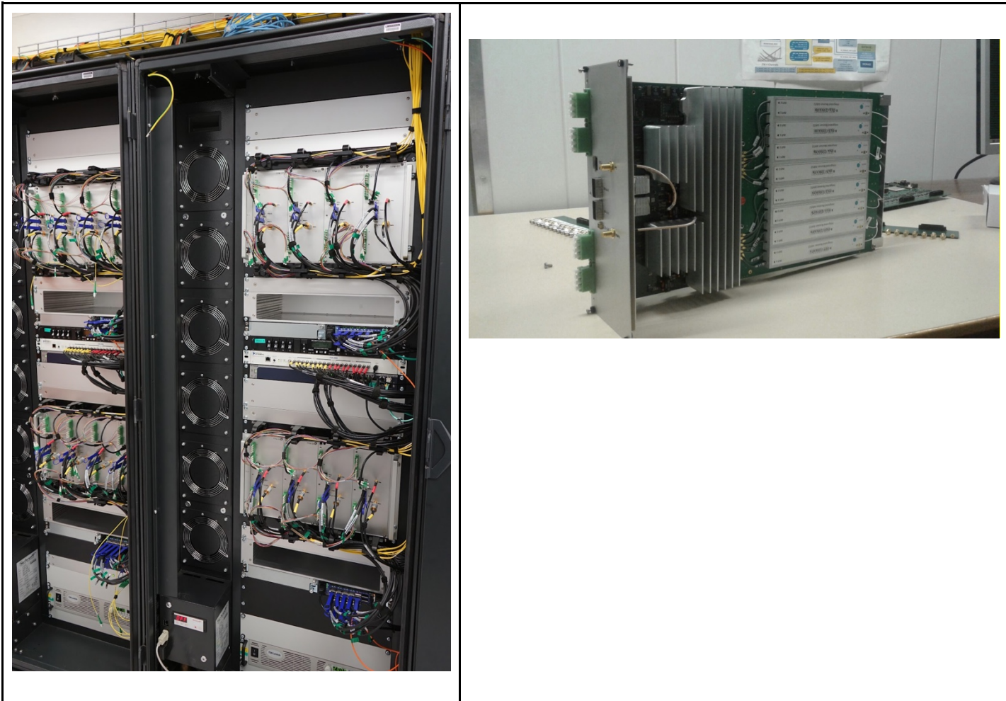
Figure 3; The Signal Processing Cabinet and a Tile Processing Module (TPM) on the right
