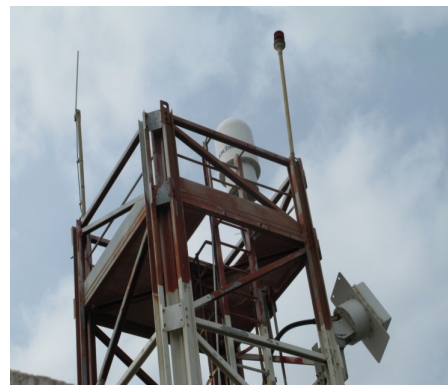
Fig. 1. The "Flight Termination System" (FTS) transmitter.
