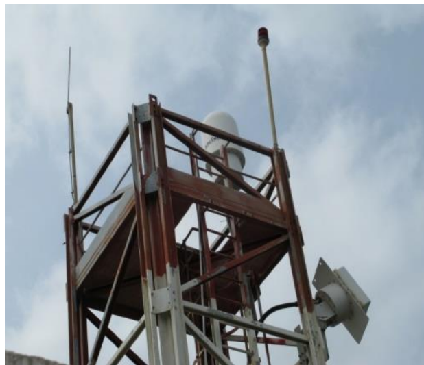
Figure 2. The “Flight Termination System” (FTS) transmitter
