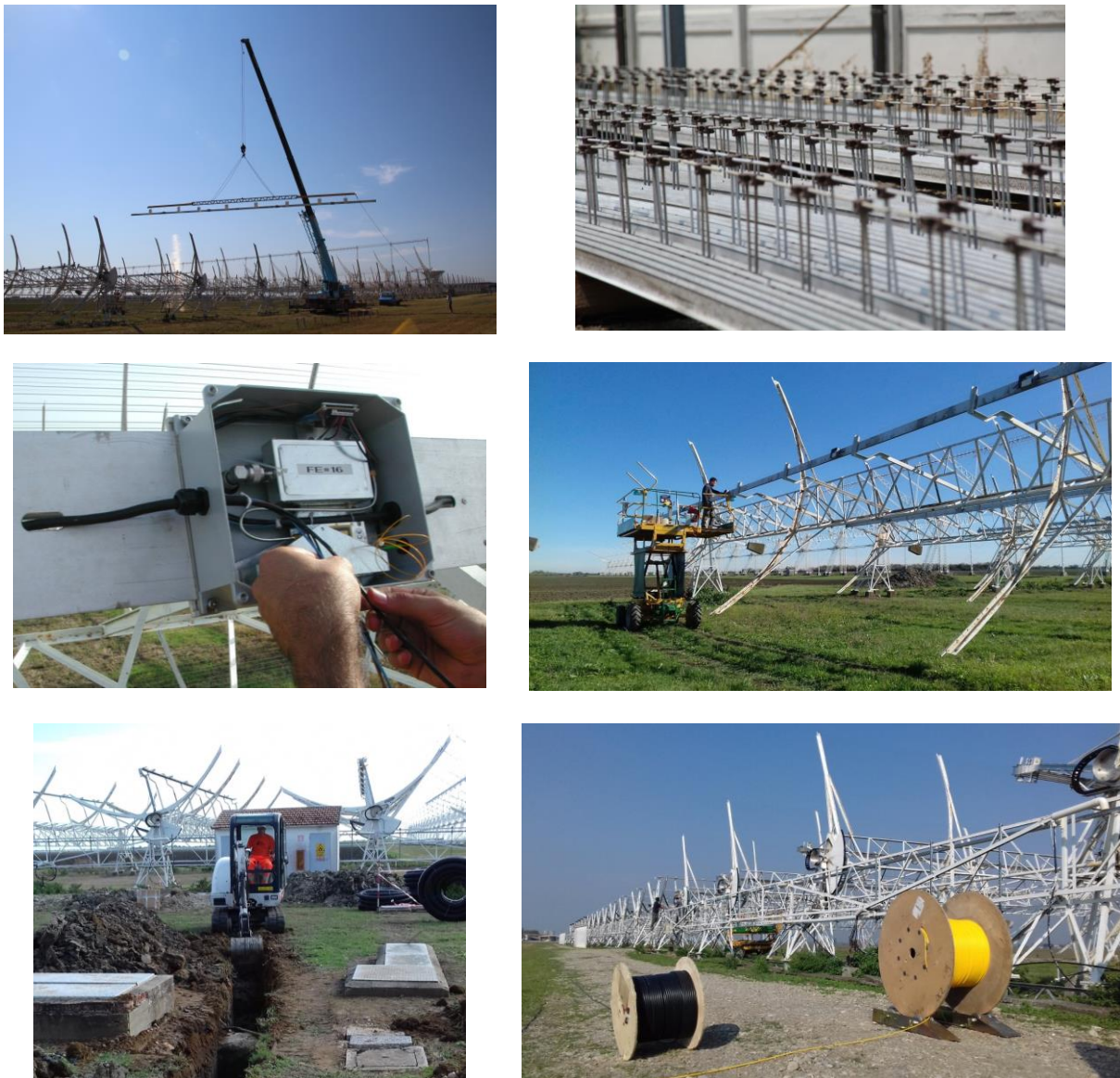
Figure 9: Upgrade of the Northern Cross antenna
