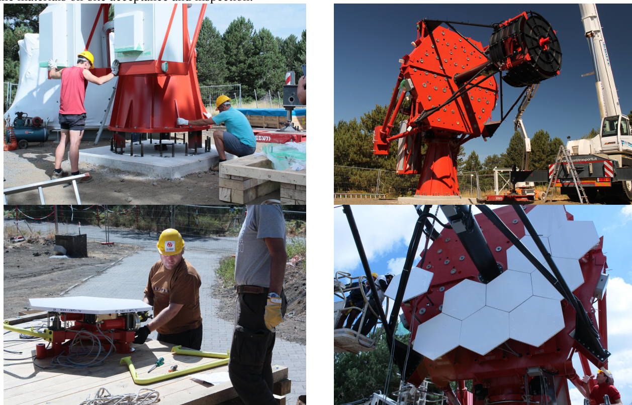
Figure 4: Highlights of the telescope opto-mechanical on-site installation. (top-left) Positioning and alignment of the mount assembly on the foundation (top-right) Completion of the telescope structure (bottom-left) Primary mirror segments and active optical support integration (bottom-right) Primary mirror installation.
