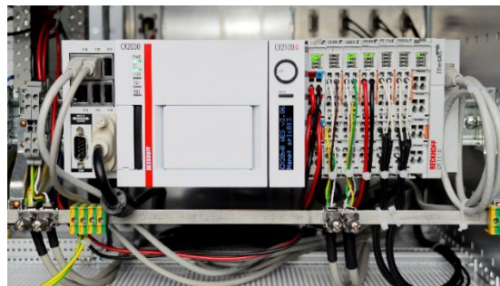
Figure 2 ESPRESSO PLC CPU#2 with functional modules
