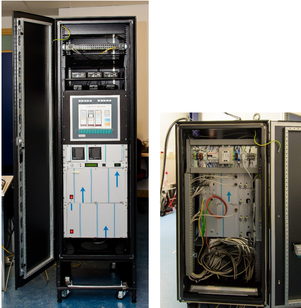
Figure 4 Instrument Main Cabinet on the left and Front End Unit Cabinet #4 on the right, both with double PLC subracks
