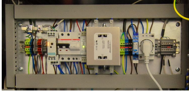
Figure 6 Electrical components in the FEU cabinets
