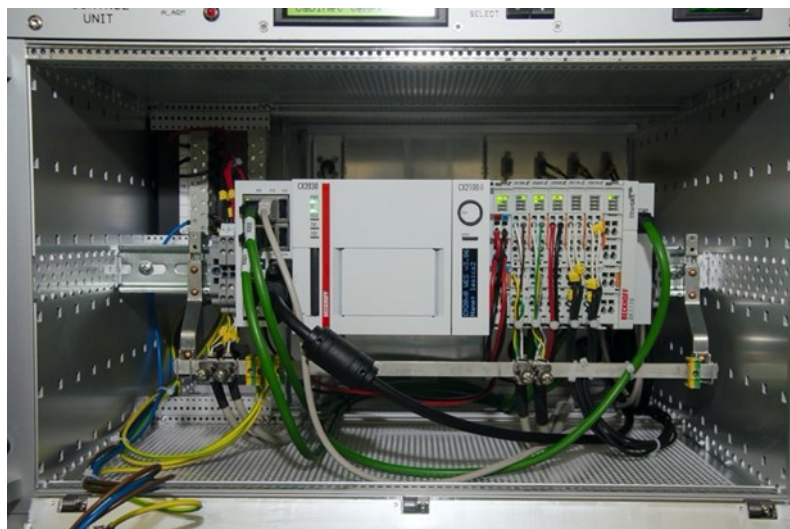
Figure 36: PLC CPU mounted in a rack.
