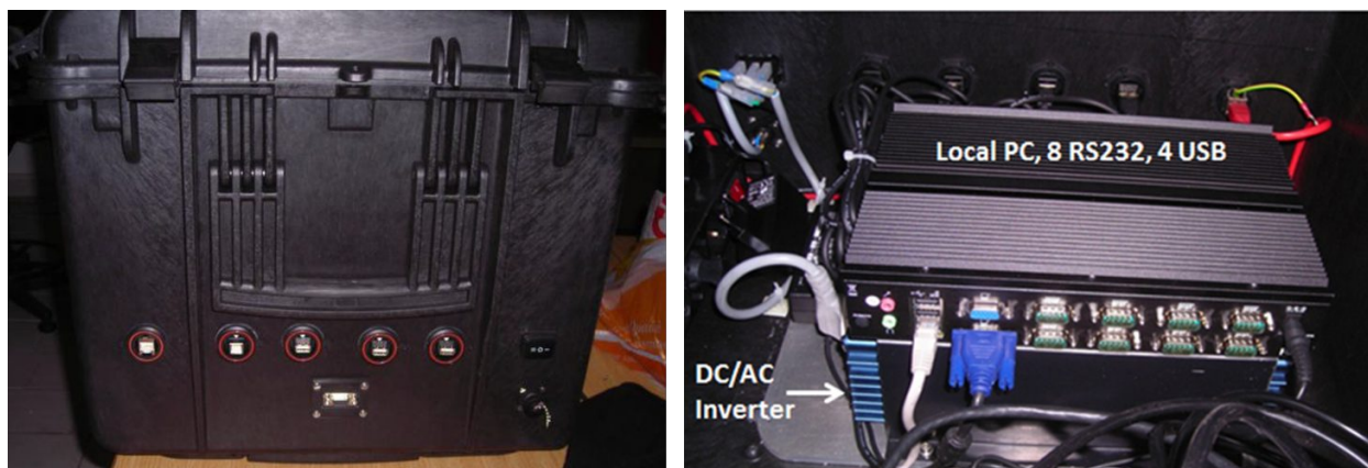
Figure 2. The Illuminator Control Box: on the left panel the exterior view showing the connectors for external interfaces; on the right panel the inside view showing the local PC used to interface and control the light generation and auxiliary devices.
