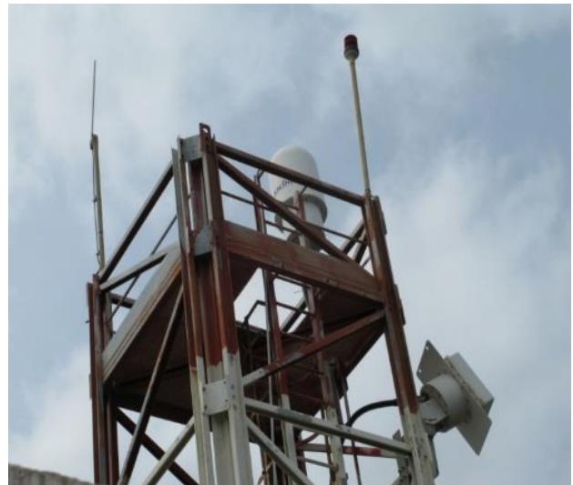
Figure 2. The “Flight Termination System” (FTS) transmitter
