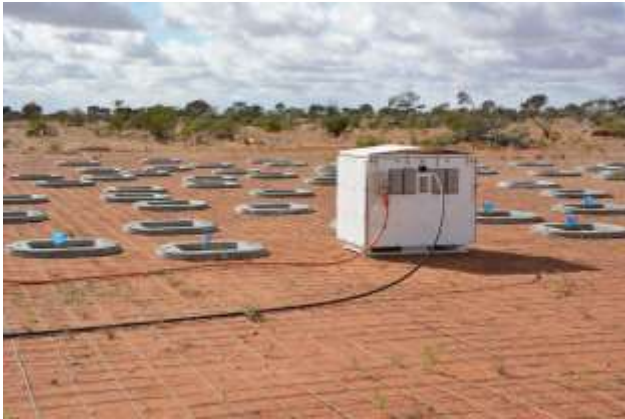
Figure 5. A section of the main station of AAVS1 showing the prepared area, ground mesh, APIU and concrete bases for the SKALA2 antennas.
