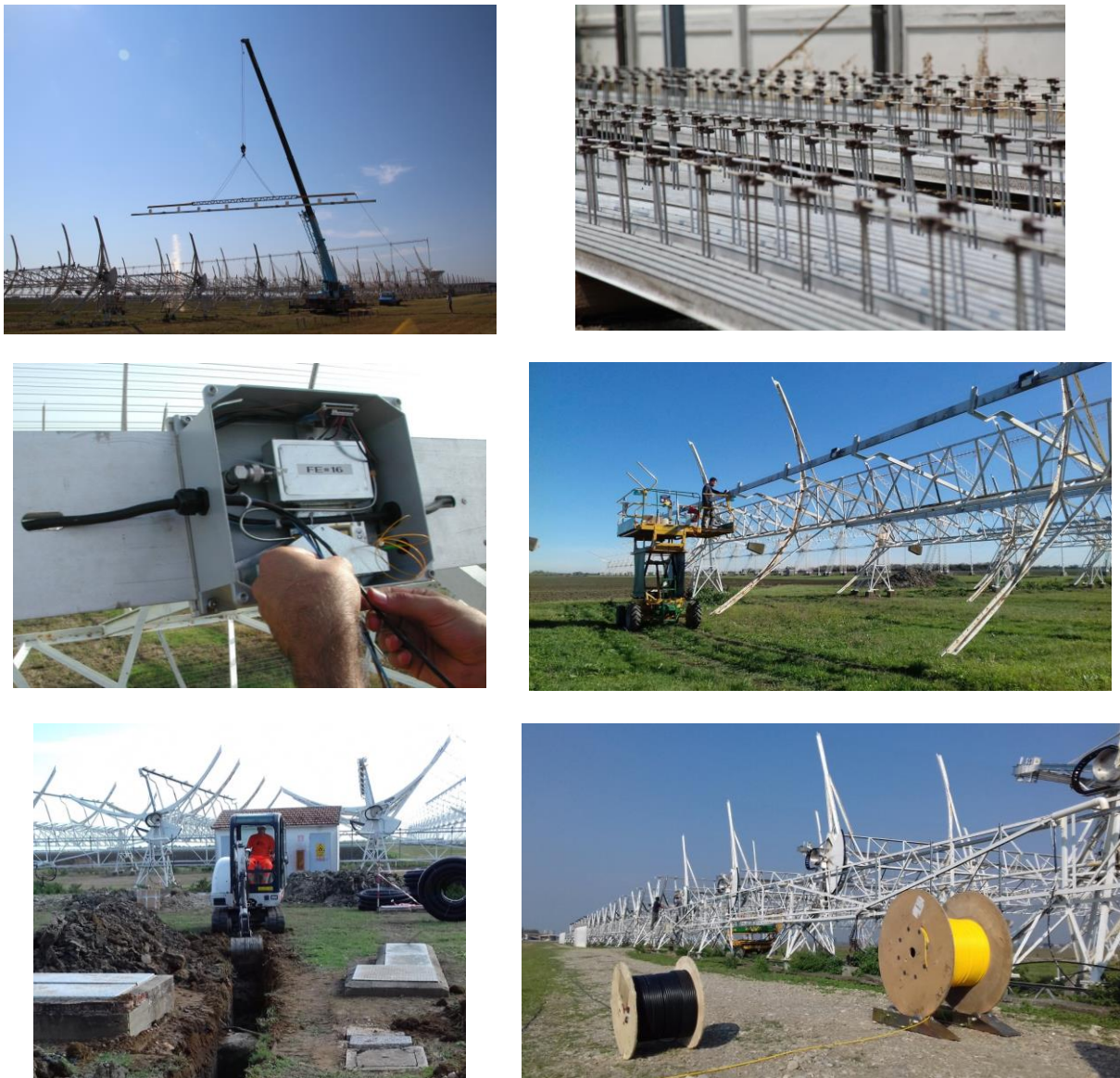
Figure 9: Upgrade of the Northern Cross antenna
