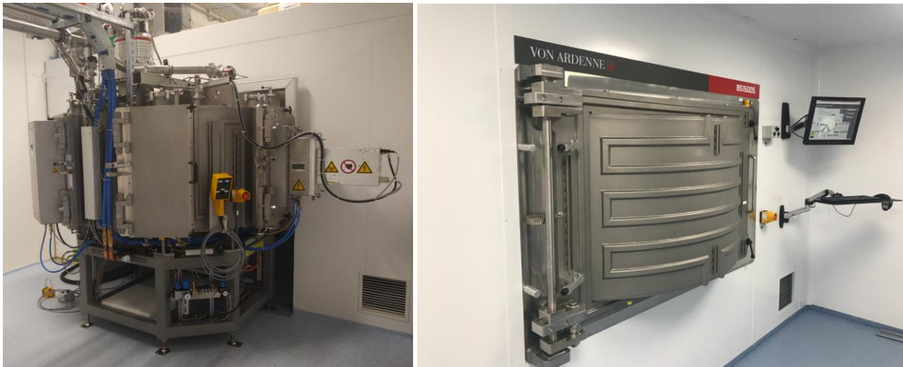
Figure 5 – Photographs of the newly installed drum coating machine for mass production of coated SPO plates. The left image shows the backside of the machine inside a grey room for easy access and service. The machine has a plasma cleaner, two magnetrons and space for a third one. The right image shows the front side of the vacuum chamber as seen from inside the cleanroom of cosine. The large door can be opened to load and unload carriers holding up to 150 SPO plates. The system is then closed, evacuated and the carousel moves the plates past the magnetrons to sputter single or multi-layers. The system is fully automated and the recipe can be set via the computer system shown in the right image.
