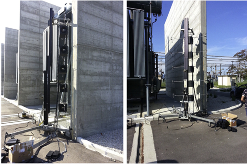
Fig. 12. Deployment of the ANC system at an electricity generation station in Tuscany (Italy).
