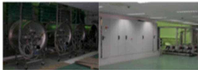
Figure 1-6: Example of cryogenic vacuum system complete of helium compressors and electrical cubicles (for reference only)
