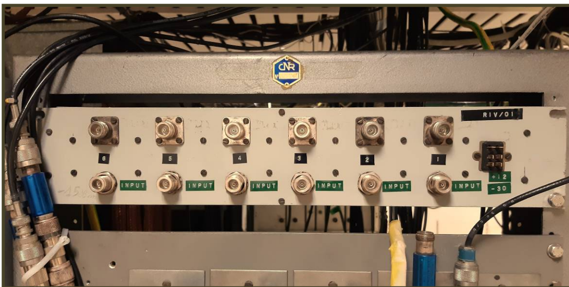
Rivelatori Ch EW – Rack 21
