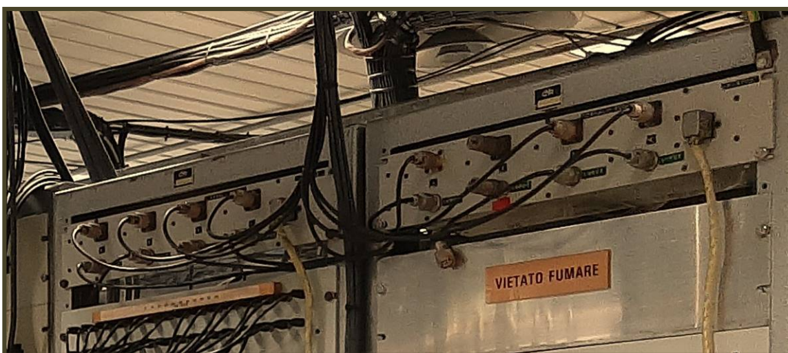
Rivelatori Ch NS – Rack 27-28
