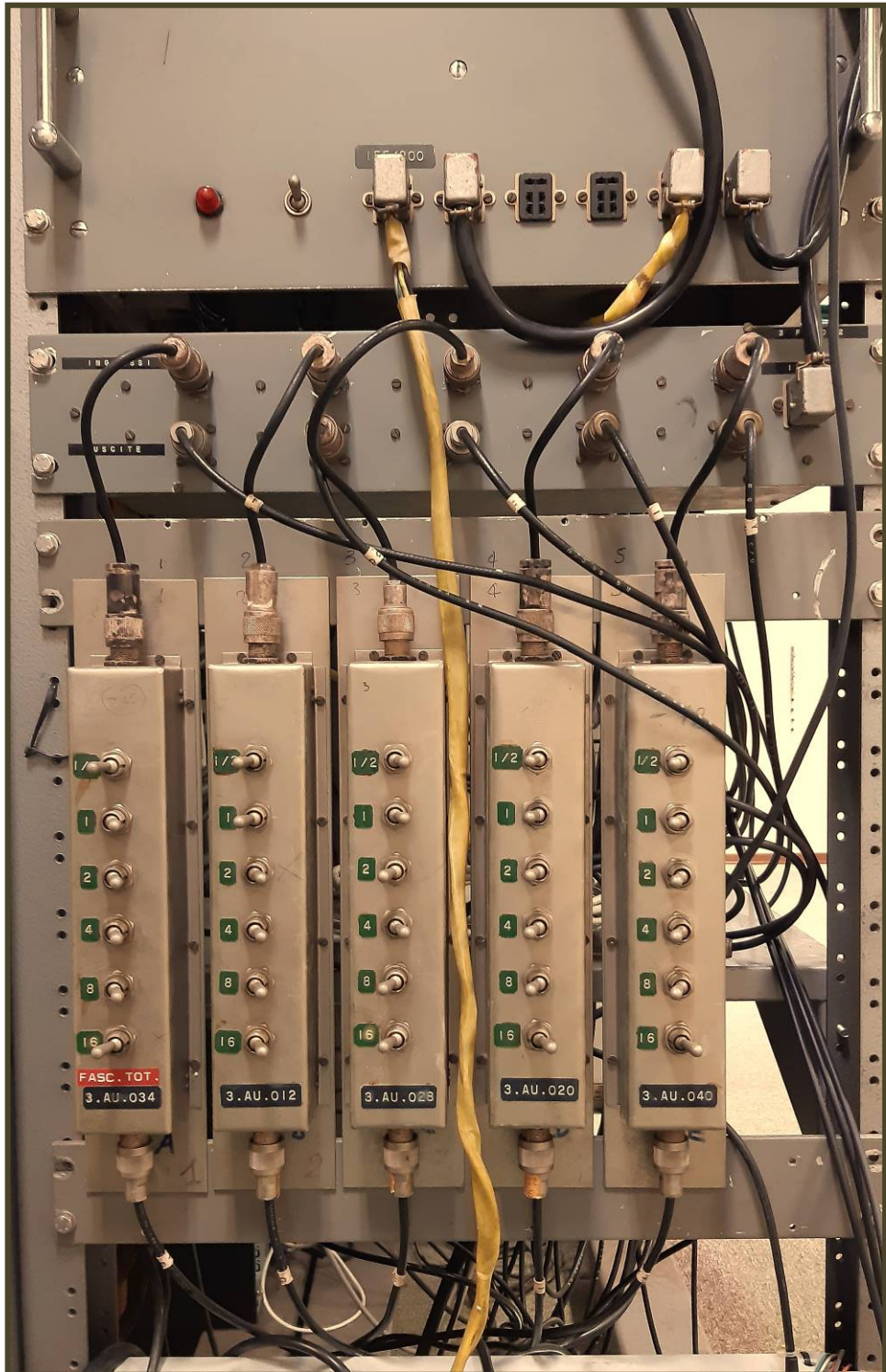
Rivelatori Fasci NS – Rack 29
