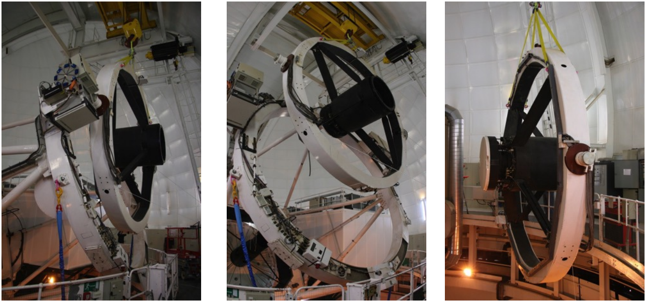
Figure 3: First trial removal of the current top-end ring as an operational test in mid-July 2016.
